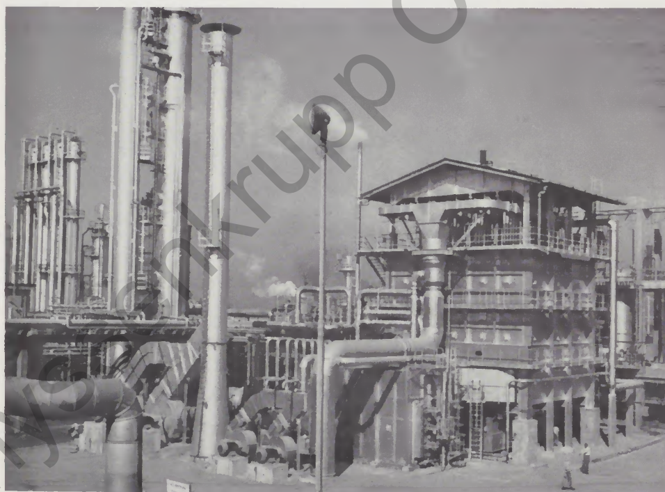
Reforming-Anlage Hindustan Steel
