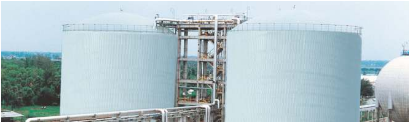
Cryogenic Ammonia Storage Tanks with associated facilities
