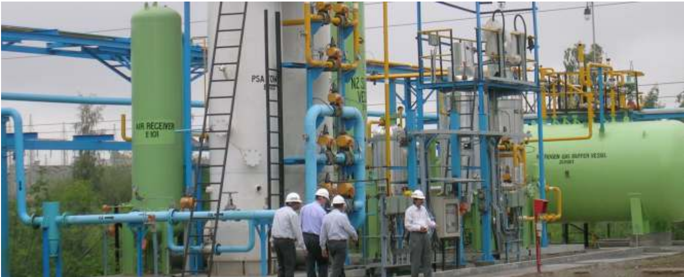
Hydrogen-Nitrogen Utilities for Steel Plant
