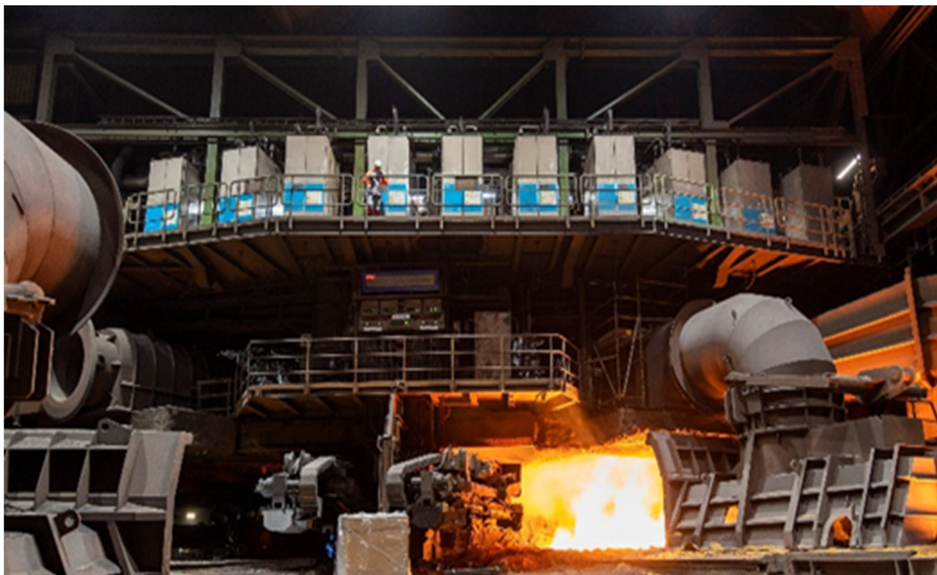
Figure 3. Image of Schwelgern BF1 SIP boxes, located on a platform above the tuyere level.
