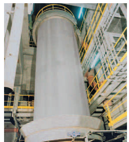
Drive unit of the fines cooler
