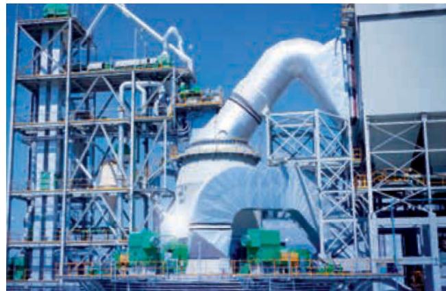
The largest QMC²-RD is installed in Mexico. The system has a rating of 4 x 1,800 kilowatt and a capacity of 300 tonnes per hour.
