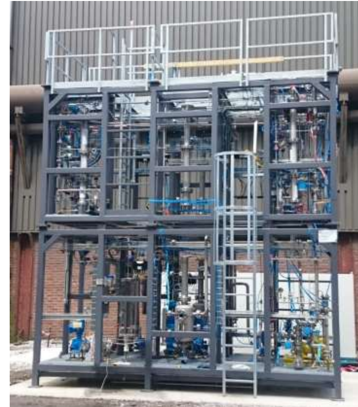
Pilot plant at thyssenkrupp Steel Duisburg Co-operation with Technical University of Berlin
