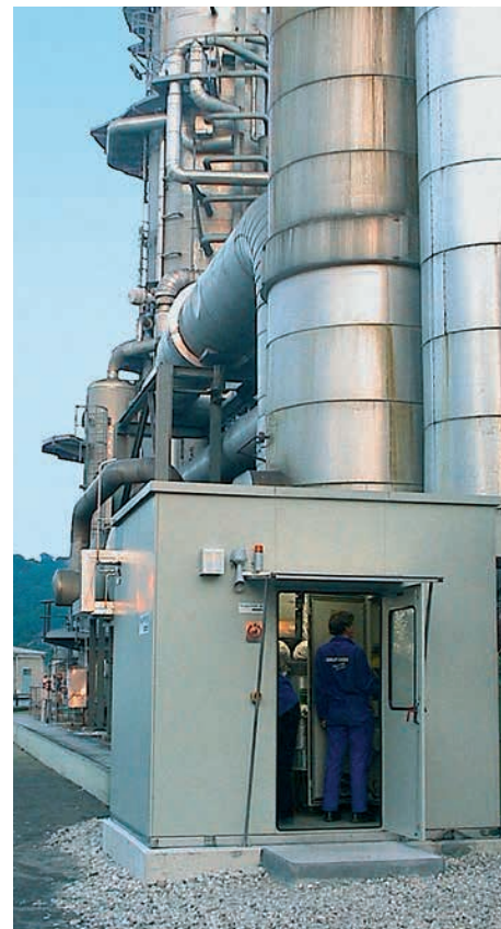
thyssenkrupp Industrial Solutions mini-plant installed at Borealis AG nitric acid plant, Austria
