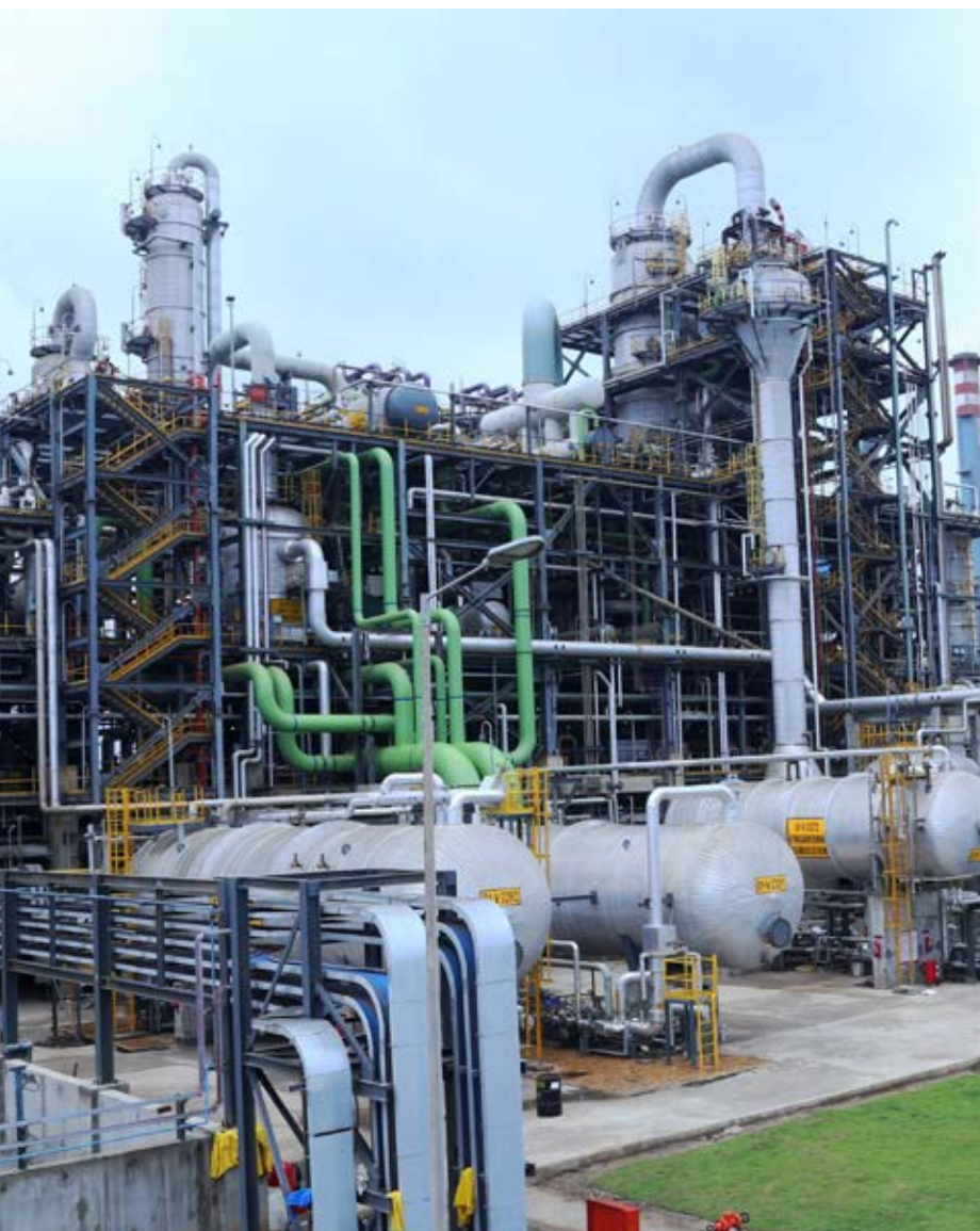
Cumene-phenol plant, Dahej, 2015–16 | Cumol-Phenol Anlage, Dahej, 2015–16
