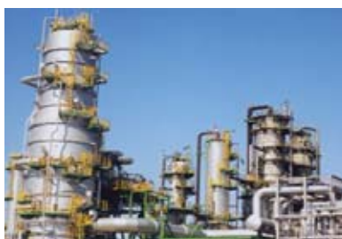
Crude oil distillation unit (Rohöldestillation) PCK Raffinerie Schwedt, Germany
