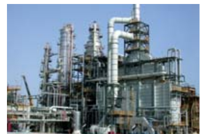
Vacuum distillation unit (Vakuumdestillationsanlage) Turkmenbashi Lube Oil Refinery, Turkmenistan
