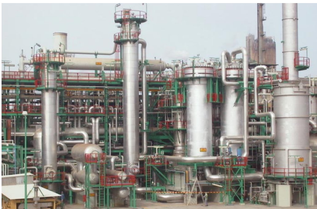
Fig. 3 | Ammonia synthesis plant, capacity 2,000 tpd, operating pressure 210 bar
