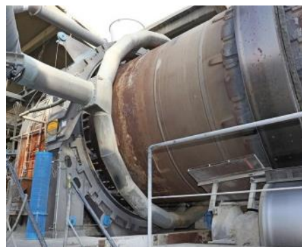
Graphite seal at a rotary kiln on the kiln outlet side.
