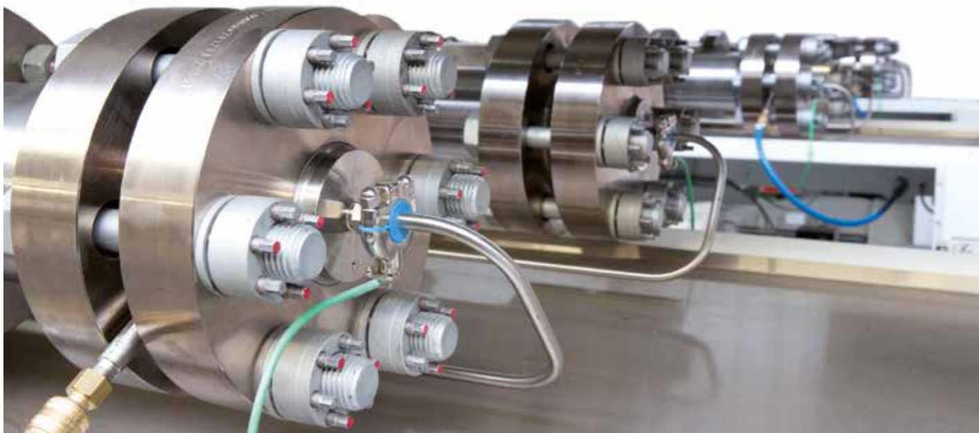
High-pressure intensifier of an HPP plant
