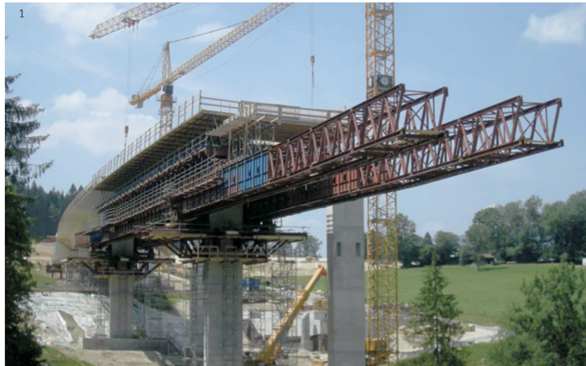
1 Construction of the new Eaux de Fontaines viaduct in the Canton of Bern, Switzerland.
