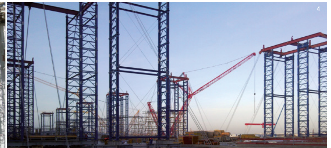
4 Berlin Brandenburg Airport, auxiliary towers for the construction of the terminal roof.
